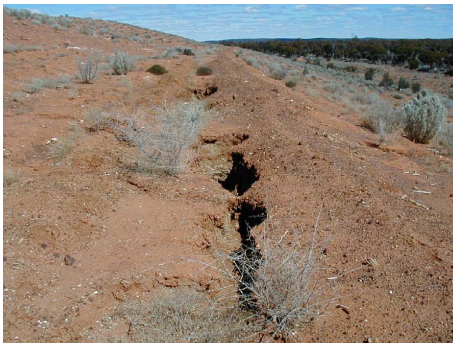
Figure 2. Tunnel development due to ponding of water in a berm on a mine waste rock dump.
